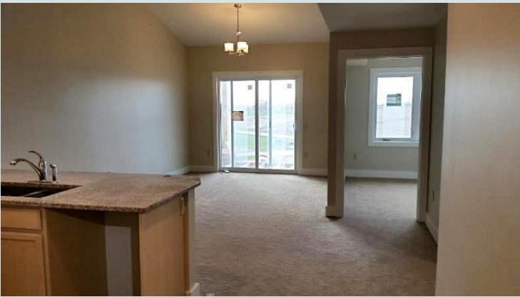
(Above Photo) Apartments are now having counters and carpet installed. The apartments are starting to look more like "home".
