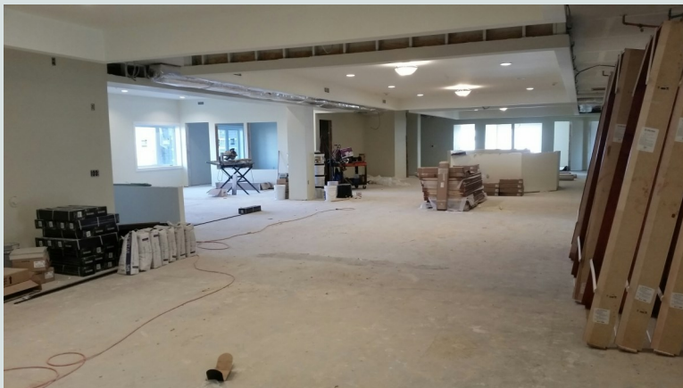
(Above Photo) Door frames and doors are being installed in the Memory care. The cherry finish really accents the doorways.
