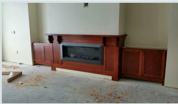
(Above Photo) The fireplace has been added to our Bistro/Lounge area. Seating will be placed in front of the this gorgeous fireplace! Just imaging relaxing in front of that!
